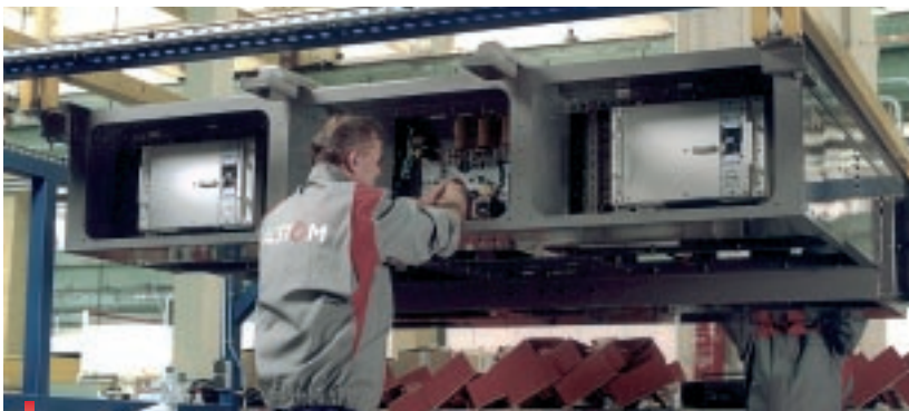
ONIX traction system prior to installation
